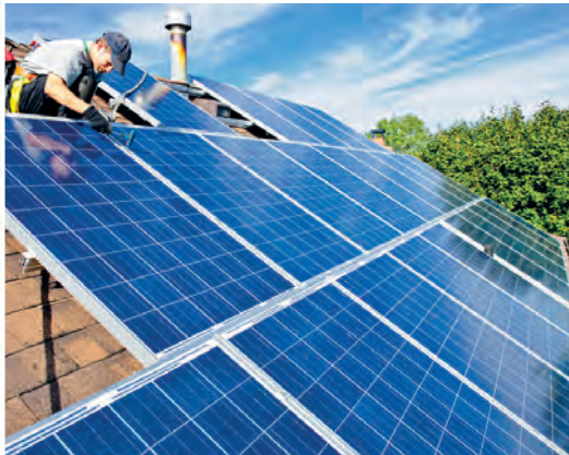
Solar Panels for Free electricity
